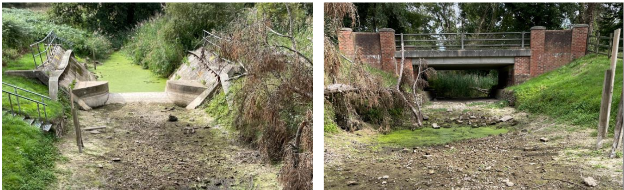
Figure 29 - Images showing dry riverbed in the month of September at Euston gauging station on the Little Ouse upstream of the Sapiston confluence during the 2022/23 drought
