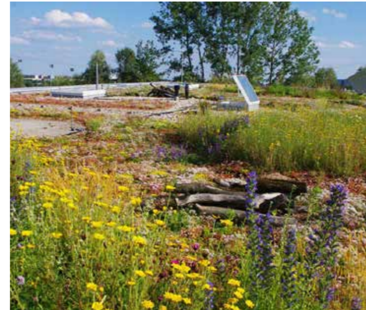
Green roof system to enhance biodiversity
