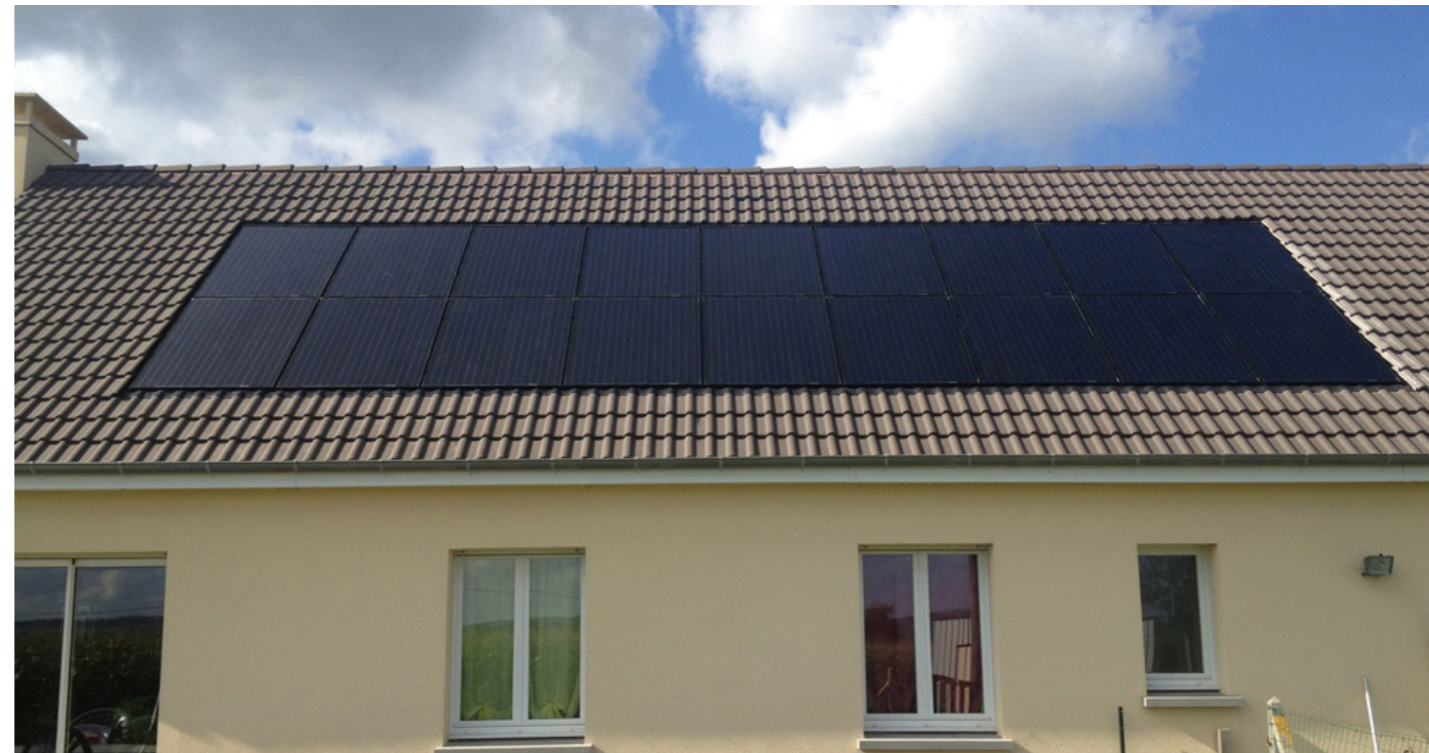
Figure 64. Roof Integrated Photovoltaic Panels
