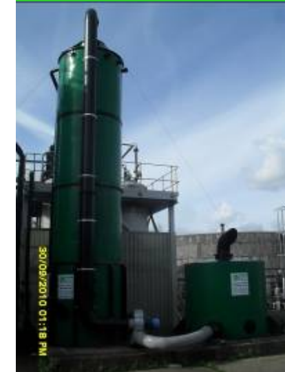
Modified Water Treatment Plant
