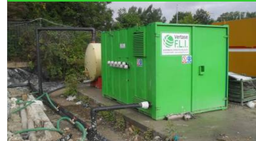
A force Ventilation Unit
