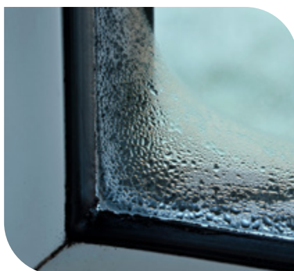
| Condensation on the inside of a window
