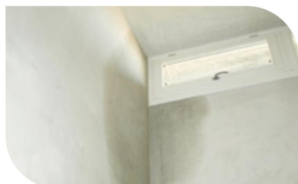
| Damp patches that need resolving
