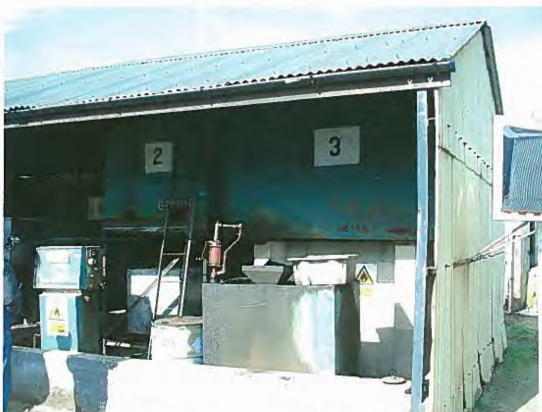
Tanks 2 and 3 used to store red diesel, pump and waste oil tank in off-site farm yard.
