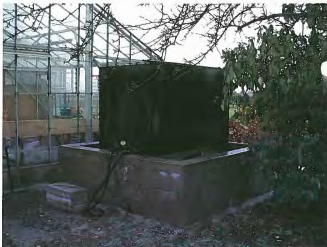
AST located beside Spore Proof Building/ glasshouse used to store diesel
