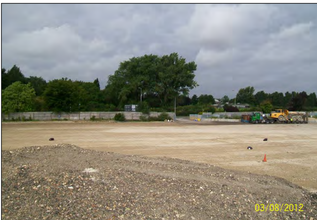
Figure 24. As built: Area of reinstatement of TB179 (retained tarmac stockpile in foreground).
