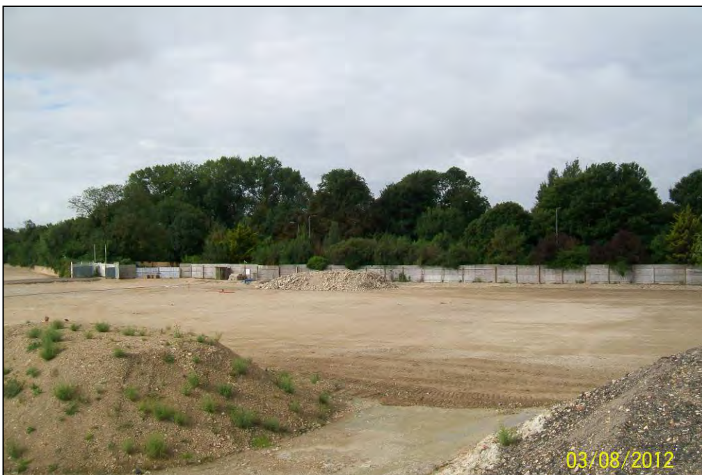
Figure 26. As built: Area of reinstatement of TB179 (retained tarmac stockpile to right, retained made ground stockpile to left, retained crush concrete stockpile (relocated) in background).
