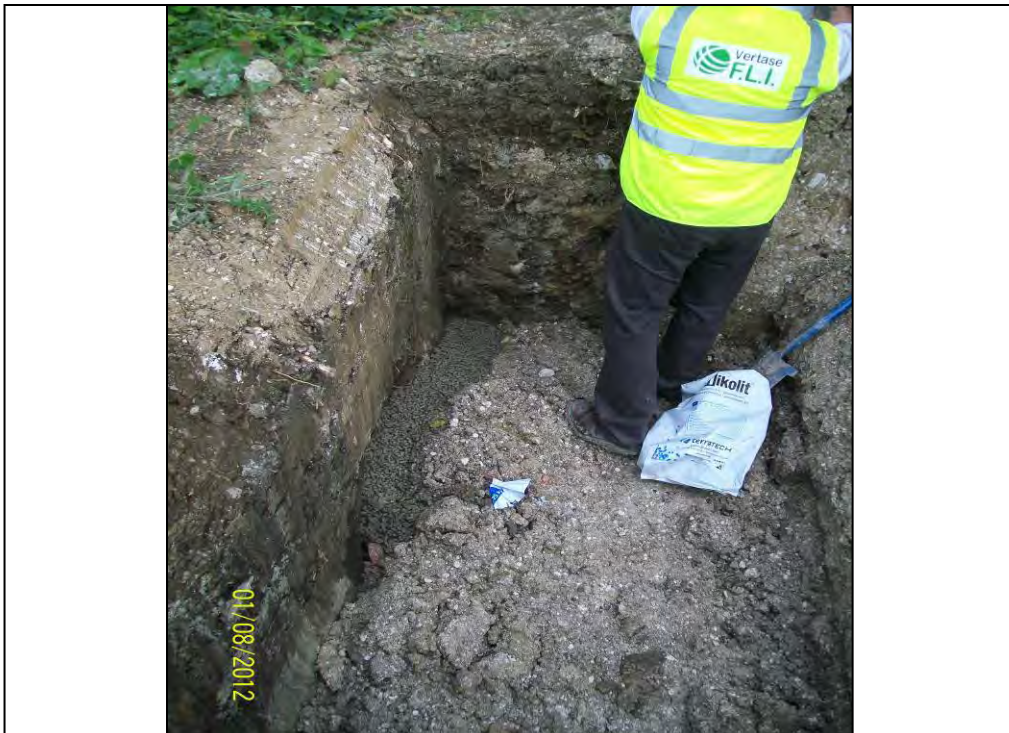
Figure 7. Bentonite plug being installed along full width of outfall pipe and pea gravel.
