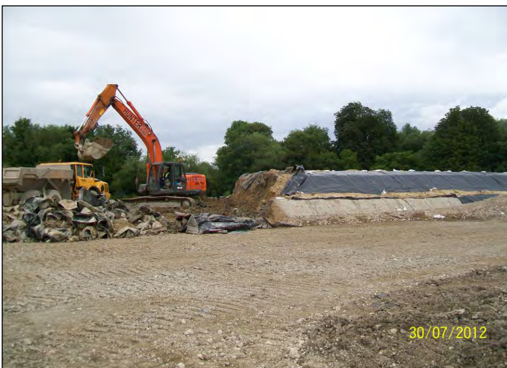
Figure 14. TB179 being loaded into dumper truck for reinstatement. Bed remained covered to face in order to control any unexpected odours.
