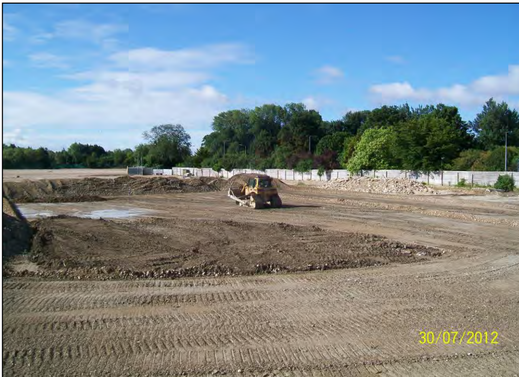
Figure 13. Caterpillar D6 grading up crush concrete to stockpile prior to reinstatement of TB179.
