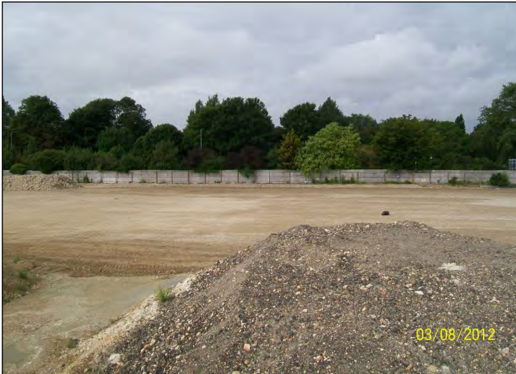
Figure 25. As built: Area of reinstatement of TB179 (retained tarmac stockpile in foreground).
