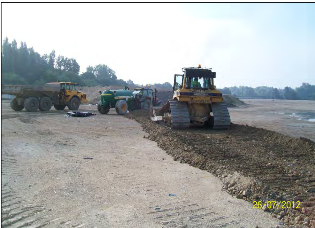
Figure 12. Caterpillar D6 grading up crush concrete to stockpile prior to reinstatement of TB179.
