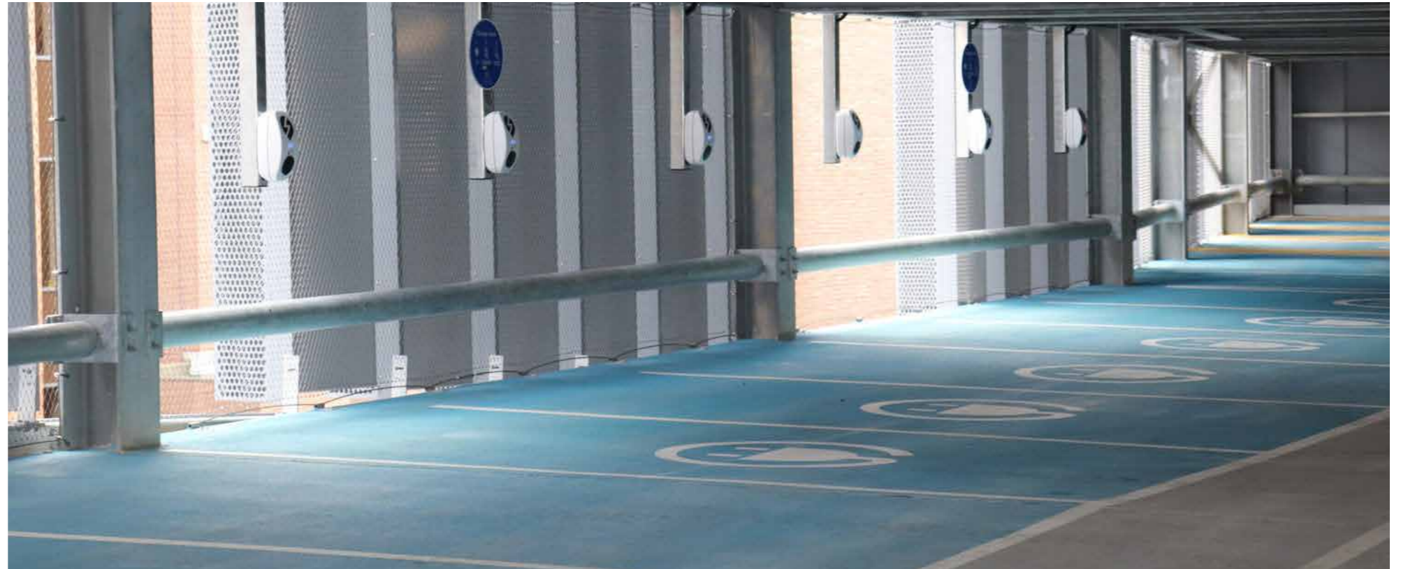
Ceiling mounted EV charging points
