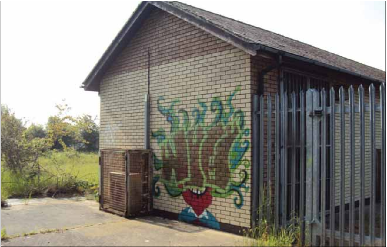
Plate 9: Existing Buildings – Signalling Relay room
